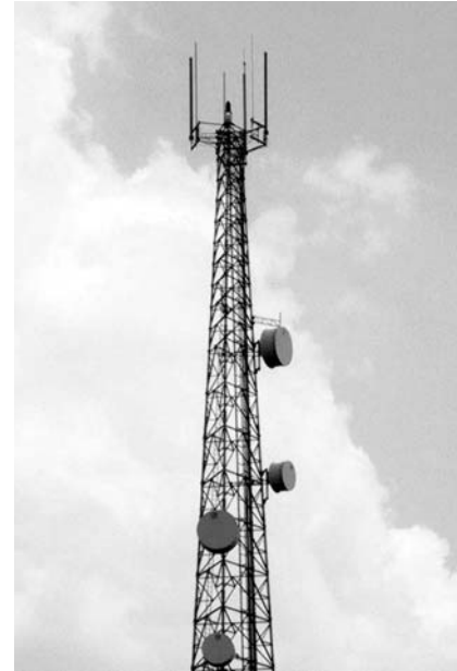
Tower with RFS Omni Antennas
