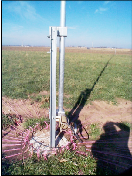
Figure 2—Titanex antenna, loading coil, radials and feed line.
